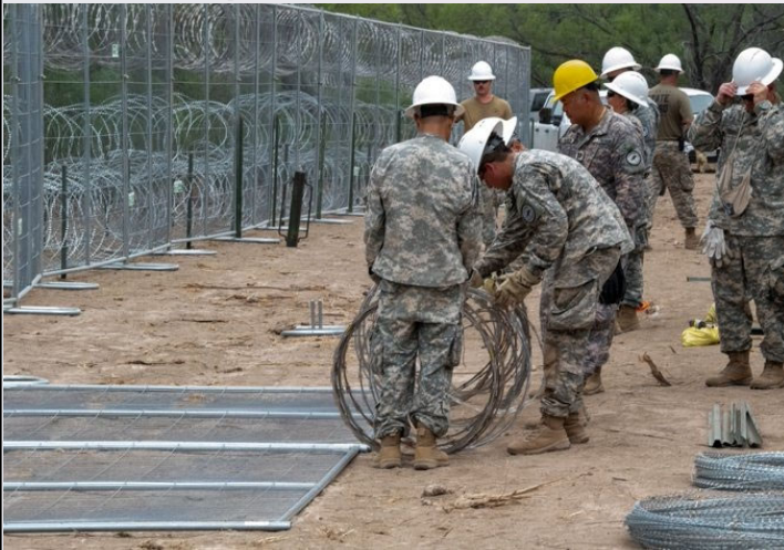
EAGLE PASS, Texas-- Florida State Guardsmen install anti-climb barrier along the Texas - Mexico border. #OperationLoneStar
